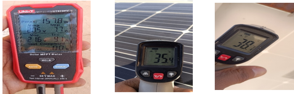
Figure 14. Solar panel output meter reading and temperature after cooling process
