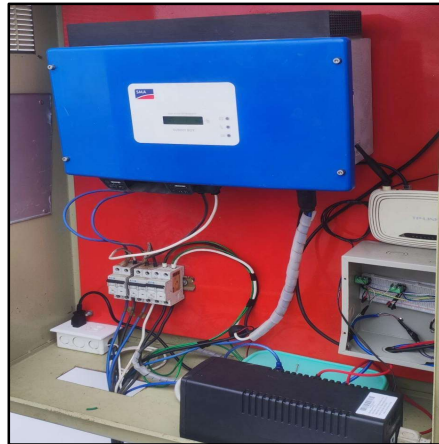
Figure 4. Location of the monitoring system components in the inverter cabinet
