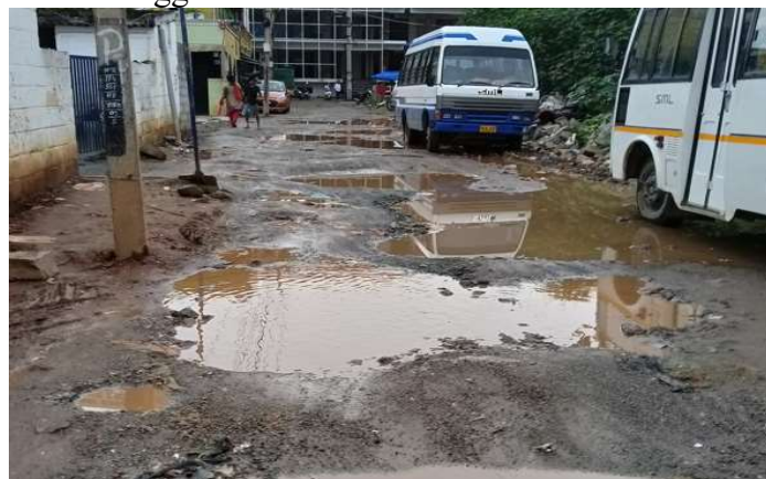
Fig 2: Suggest route has bad road condition
